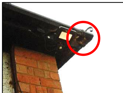
Plate 4: photograph showing a rotted crevice in the soffit located next to the flood light.
