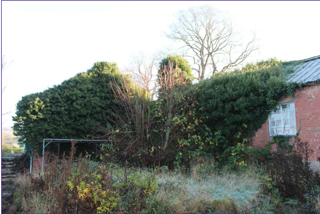
Plate 13: Heavy unmanaged vegetation growth over changing room extension.
