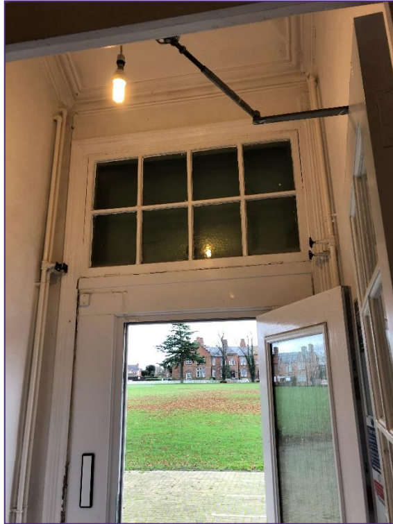
Plate 17: Original front door architraving seemingly infilled with later PVCu door casing and smaller door. Blocked off glazing above (Photo courtesy of Greenwood Projects).
