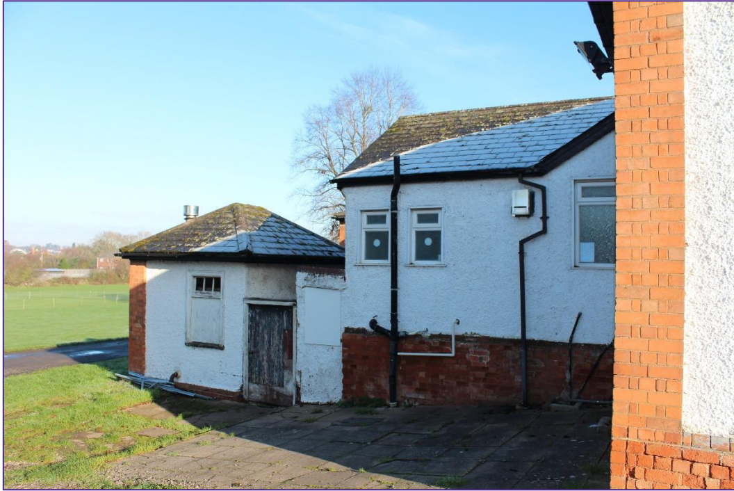
Plate 11: The west flank of the Clubhouse with earlier link-detached building noted (left). Evidence of blown brick noted on rear wing by rainwater goods.
