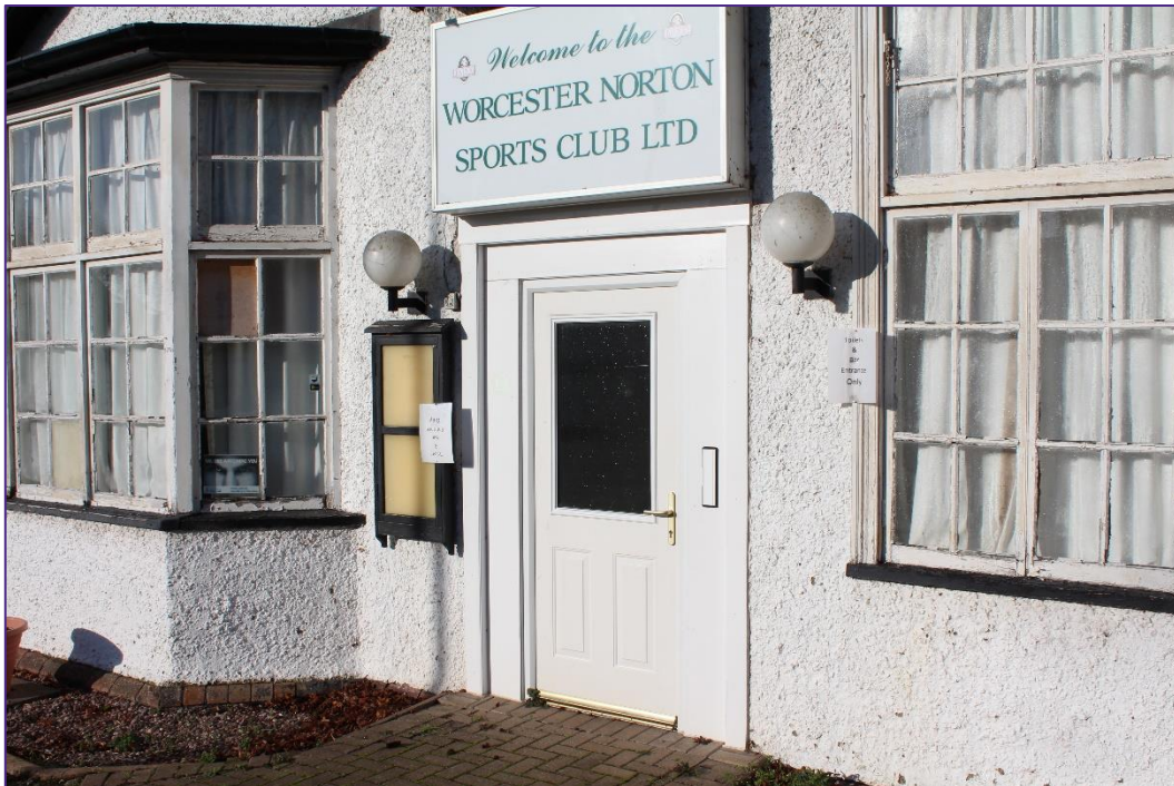
Plate 10: Later front door with heavy PVCu architraving and signage concealing original top hung casement window.
